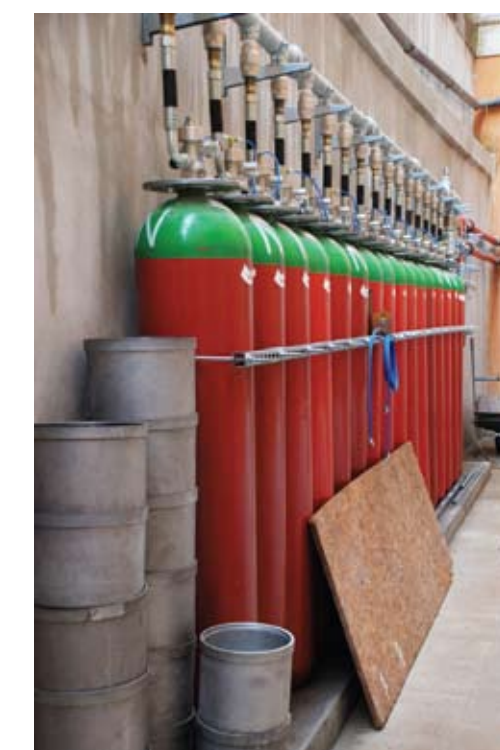
Gas tanks for new fire suppression system.
